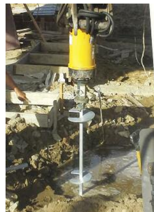
High Rise Industries: Your trusted source for certified Helical Pile Foundation System installations.
