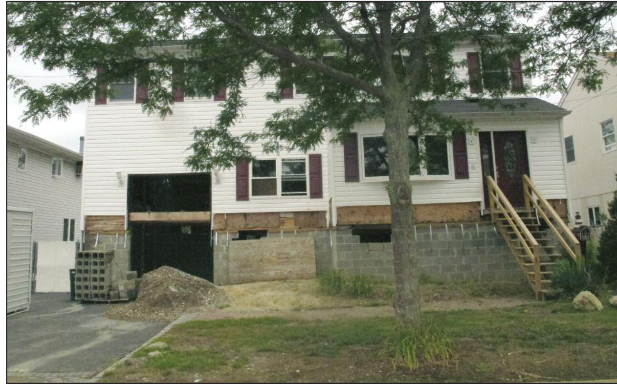
Oops! Trouble on the job site. A contractor was accused of dropping this house, which led to rapid legislation in Suffolk to ensure enough contractor liability insurance.
